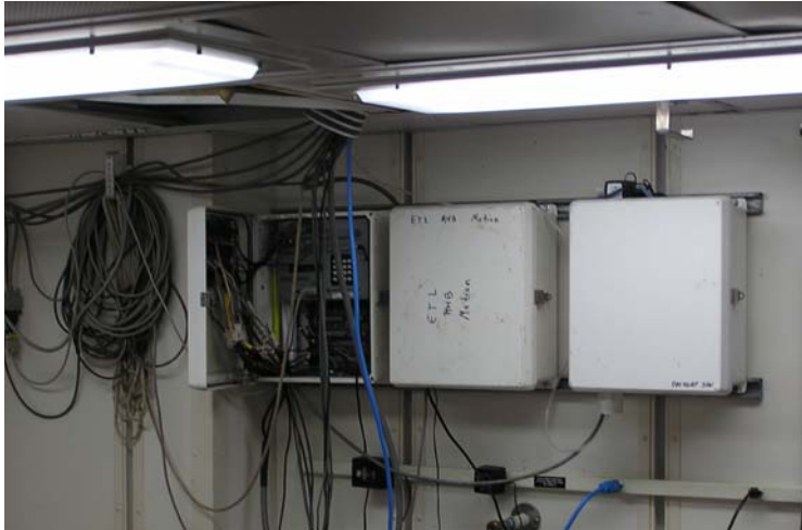
Data loggers in main computer room
